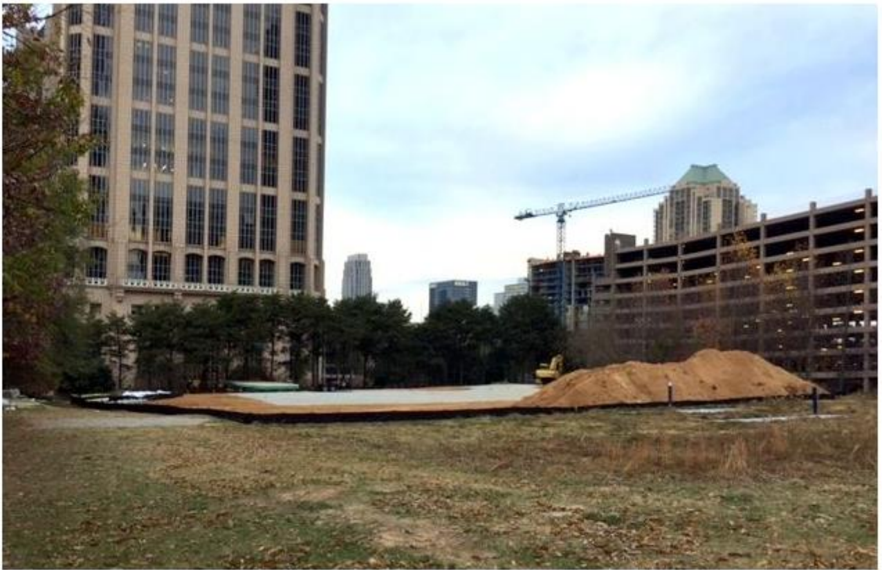
What appears to be site work at the location in question. | Carol Payne
